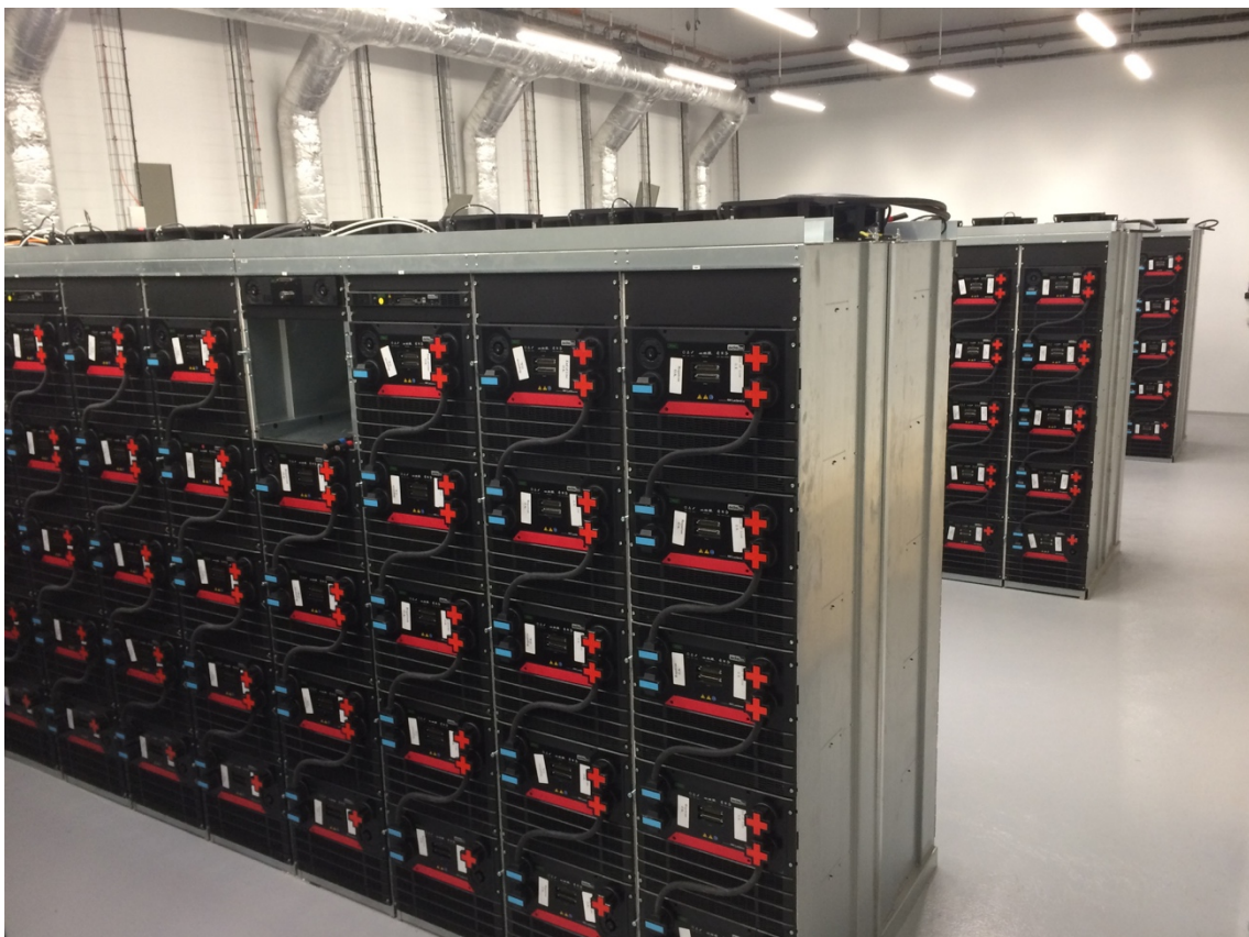
Figure 14: Battery rack at Yunicos 2.6 MW battery system on Gracioca Island
